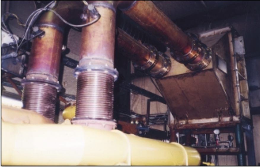
RJM Corporation's ARIS urea-based injection system installed in the exhaust gas stream (foreground) and the Johnson Matthey catalyst (background).
