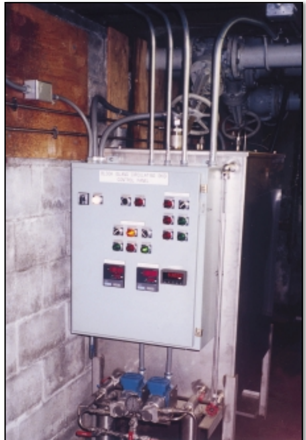
Urea storage tank, circulation skid and control panel for the utility's emission reduction system.
