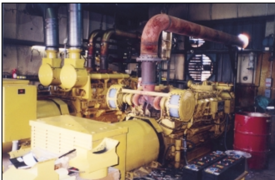
Two of four Caterpillar diesel generator sets situated in the main power generation building of Block Island Power Company. A small island dominated by its summer tourist trade, Block Island usually sees peak summer demand reach 3350 kW. The utility, therefore, has installed an additional 1300 kW Cat 3516B-powered gen-set to help ensure power availability on the island.
